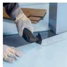
Cutting sound dampening panels, rubber mats, carpet, etc. to size cleanly and efficiently
